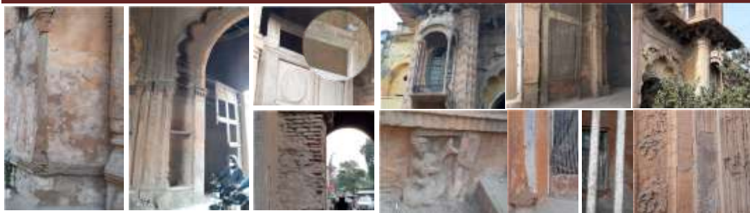
Fig-7 Lakhidarwajas in dilapidated state.
