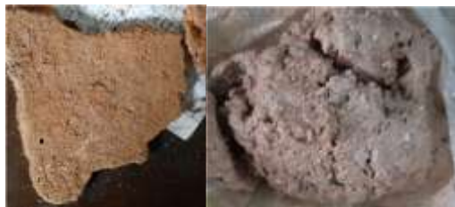
Fig-3 a) weathered lime-stucco collected from Kothi Roshan-ud-Daula b) New plaster prepared for restoration
