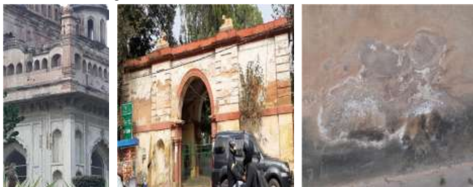
Fig. 4 a) Makbara Saadat Ali Khan; black crust and flaking of plaster exposing lakhauri bricks b) Neil's Gate; visible colour change, loss of plaster as powder c) Tomb of Mushir Zadi; Flostectorii degradation by Actinobacteria
