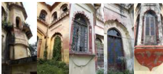
Fig-5. PariKhana: visible change in colour, detachment of parapet, crack formation with plants
