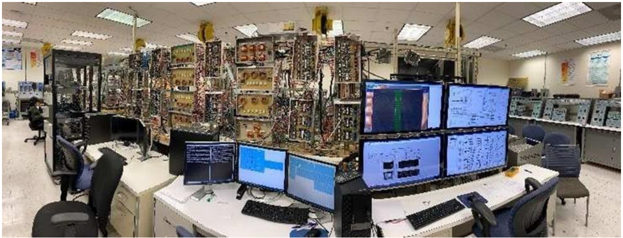
Figure 1: Smart Grid Testbed in Energy Systems Research Laboratory
